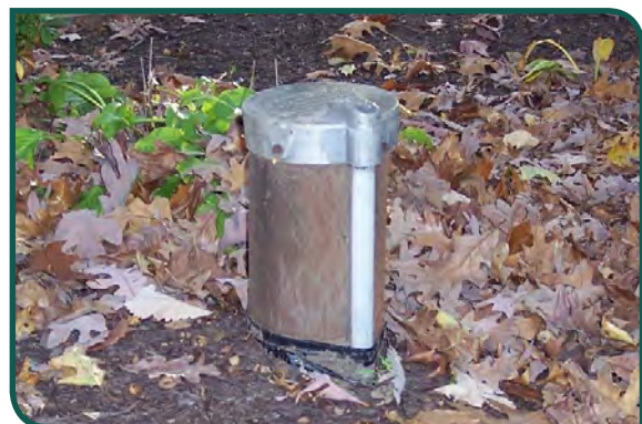
Private wellhead in residential neighborhood, Carroll Valley Borough
